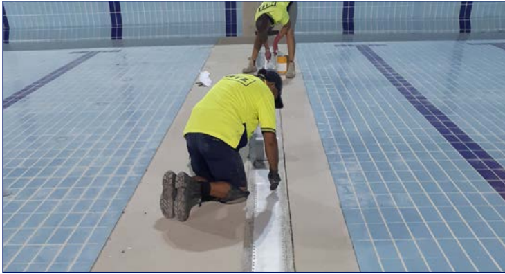
Installation of waterproofing bandage at a major construction joint. This critical work requires experience, an attention to detail and professional supervision to oversee installation.
