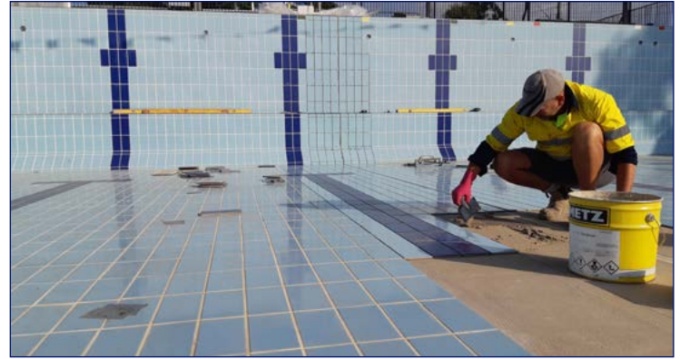
Infill tiling after installation of a properly detailed and constructed waterproofing bandage at a major construction joint.
