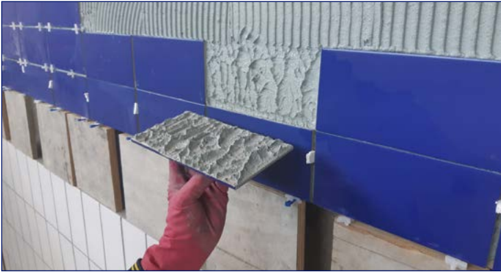
Regular quality checks are required to ensure complete adhesive coverage is obtained when tiling commercial pools. Inadequate adhesive coverage is a common contributor to tile adhesive failures Metz is called to rectify.
