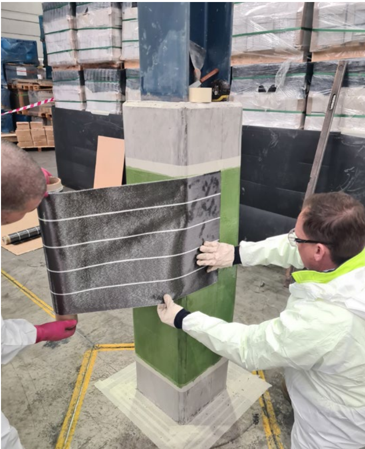
The carbon fibre fabric is unrolled into the still wet impregnating resin Metz C100
