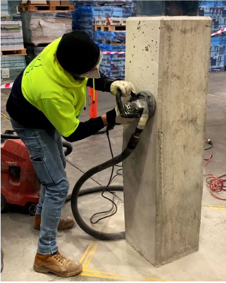
For concrete the process involves grinding, rounding corners, filling holes and smoothing
